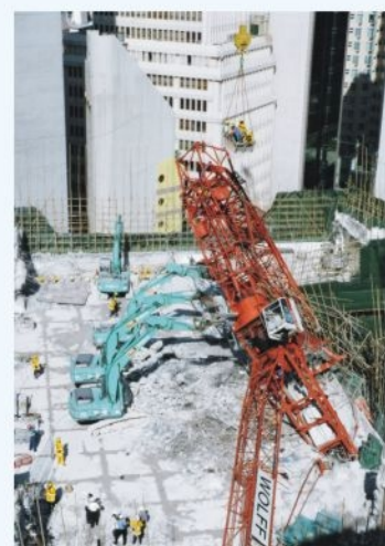
● 消防及救護人員在天秤倒塌地盤進行拯救工作 Firemen and ambulancemen carrying out rescue operation in a tower crane collapse incident
